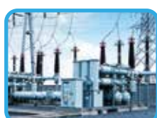
Electricity Generation and Distribution
